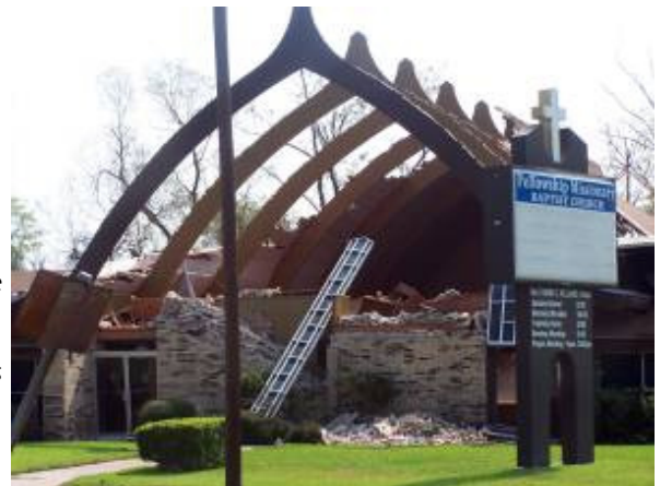
Church in Beaumont with roof ripped off by Hurricane Rita. Photo by Steve Buser.
