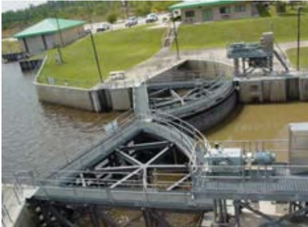
Boat Pass at the LNVA Saltwater Barrier
