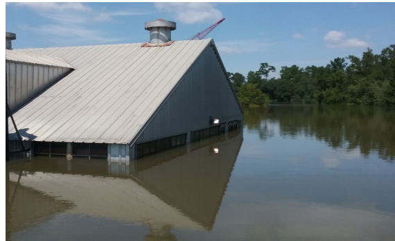
LNVA Neches 1st Pumping Station flooded by the Neches River.
