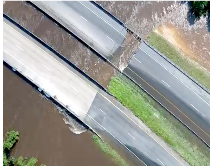
Bridge approach washout on Hwy 96 near Village Creek .
